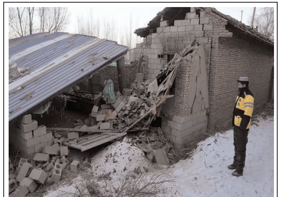
A resident looks at a collapsed shed in Yangwa village near Dahejia town in northwestern China's Gansu province. A strong overnight earthquake rattled a mountainous region of northwestern China, authorities said Tuesday, destroying homes, leaving residents out in a below-freezing winter night and killing many in the nation's deadliest quake in nine years.
